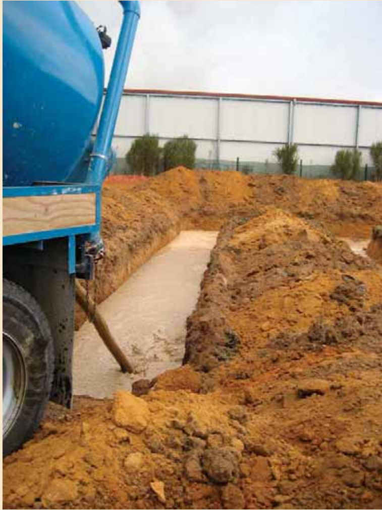
Figure 23: Sucker truck discharges into trenches dug in paddocks adjacent to Icepak facility
